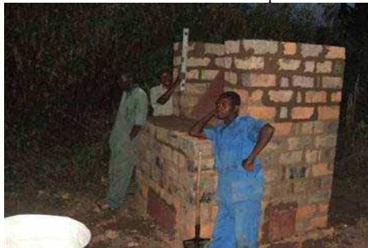
Incinerator for Lubondaie Hospital
